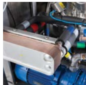
Multi-colour coded piping with isolation
